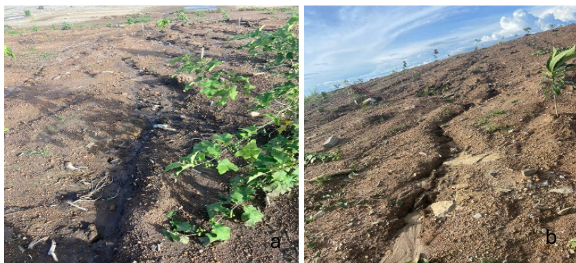
Figure 13: Visible erosion effect on restored sites: (a) in zone A and (b) in zone B
